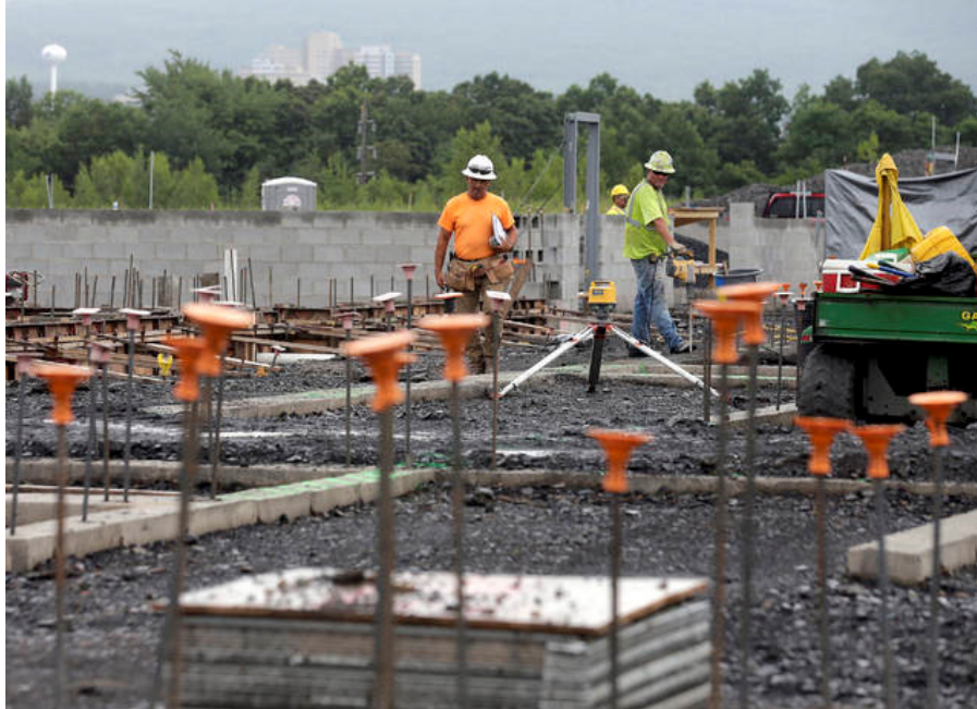
Pictures Work proceeds among foundation footers with reinforced bar jutting up to support concrete masonry unit walls — like those partially completed in the background — at the construction site of WB Area’s consolidated high school. Bill Tarutis | For Times Leader
