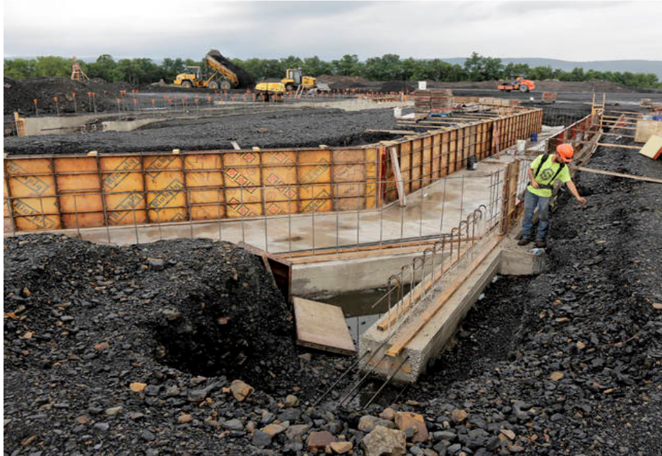
The front of the auditorium stage is outlined as workers continue construction of Wilkes-Barre Area's new consolidate high school. Bill Tarutis | For Times Leader
