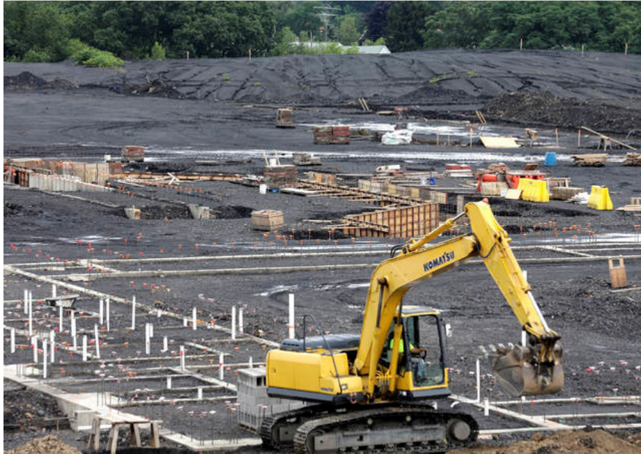
Workers have begun building concrete masonry unit walls at the site of the Wilkes-Barre Area consolidated high school. Foundation work is well underway at the construction site of Wilkes-Barre Area's consolidated high school. . Bill Tarutis | For Times Leader
