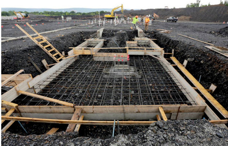
The base of an elevator shaft awaits concrete pouring on the construction site of Wilkes-Barre Area's consolidated school. (Mine Shaft High) Bill Tarutis | For Times Leader
