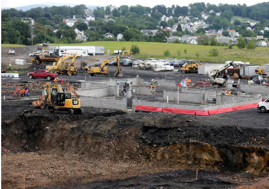
Construction continues on the swimming pool, front, in the athletic wing of the new Wilkes-Barre Area High School in Plains Township . Bill Tarutis | For Times Leader
